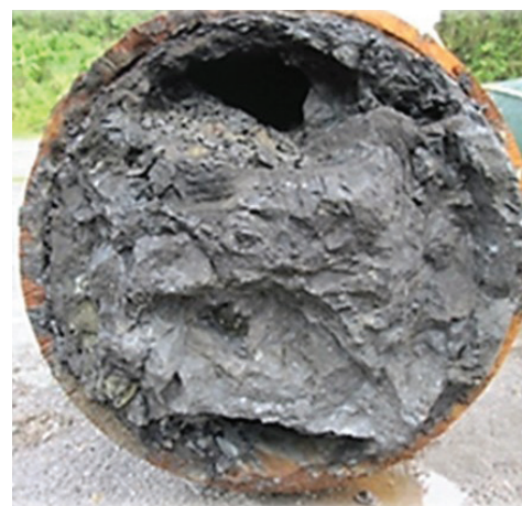
Figure 1. Mineral deposition along the 24-inch two-phase header after more than six months.
