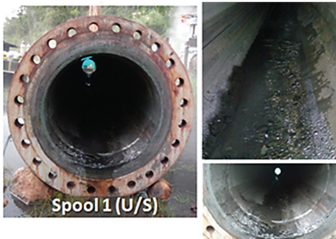
Figure 3. Visual inspection of the 24-inch two-phase header after four months of dosing.
